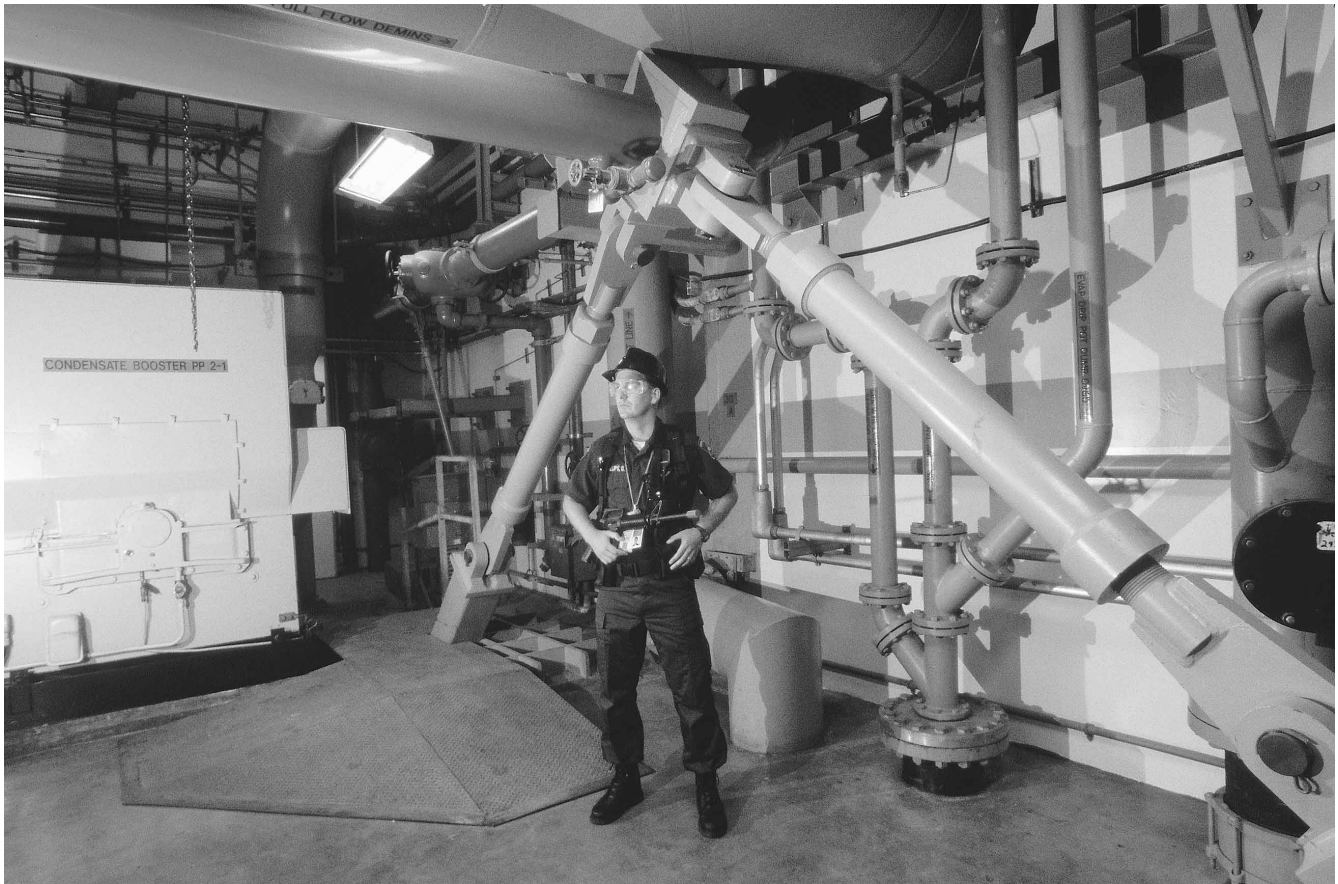
The seismic braces seen here in the Diablo Canyon Nuclear Power Plant reduce the risks associated with an area prone to earthquakes. (Corbis Corporation)
