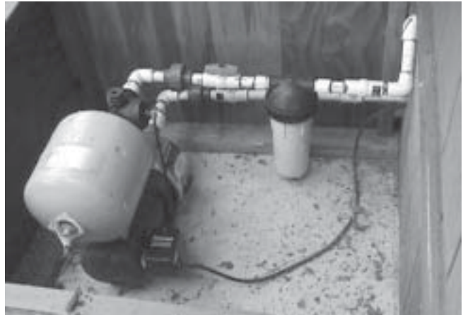
A small but typical electric pump. The pump sits below a pressure chamber. A coarse filter hanging from the inlet pipe filters the water before it enters the house.
