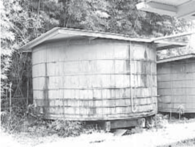
An older redwood tank. Beware of redwood tanks that were painted on the inside with lead paint to discourage algae.
