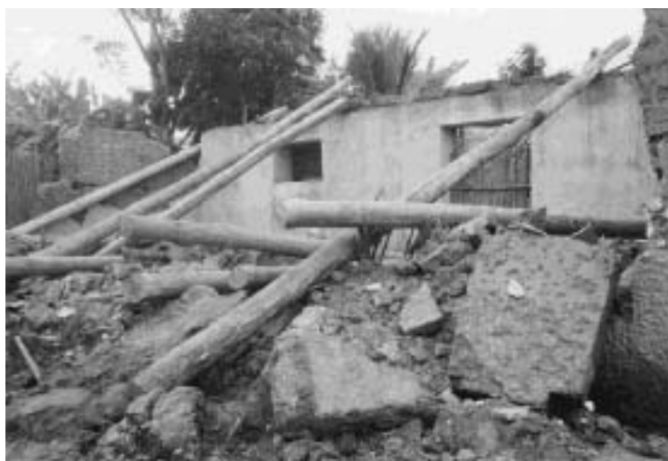
Figure 2: The impact of the earthquake on a tapial house in Soritor © ITDG/Megan Lloyed-Laney
