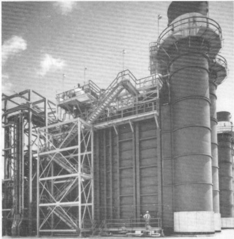
FIGURE 9.8 Heat-recovery steam generators for a cogeneration facility at Texas City, Tex., operated by Enron Power Corp., a subsidiary of Enron Corp.
