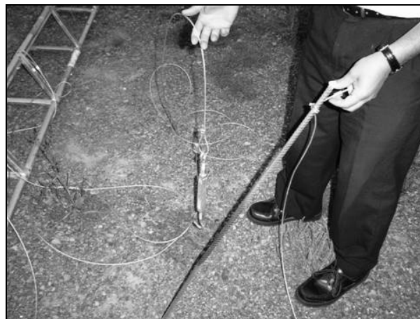
Photo 13-1: Guy Wires and Turnbuckle
