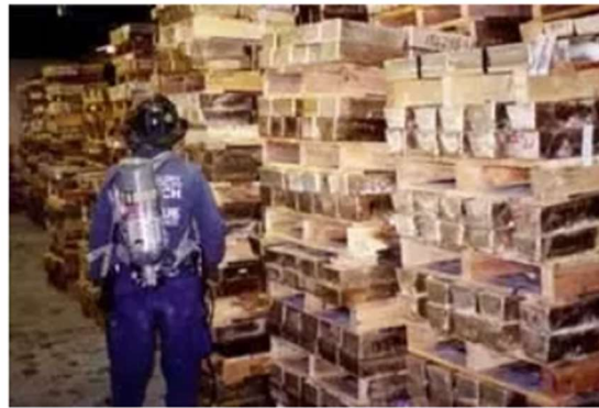
The Bank of Nova Scotia gold vault, located under WTC Building 4, is examined in late October 2001. [Source: Leslie E. Robertson and Associates]
