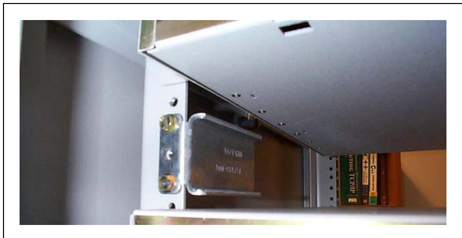
Figure 80 Installed rack-mount bracket
