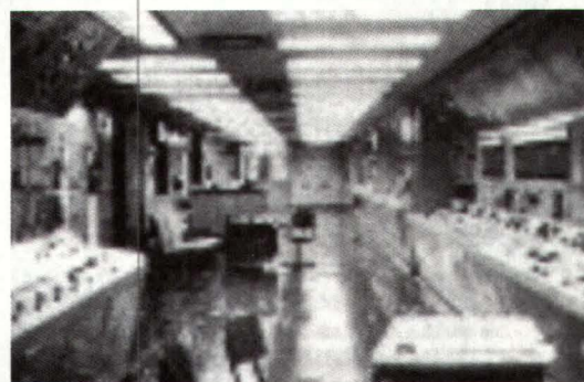
Photo of Dimona's plutonium separation control room, with equipment. Recognisable by nuclear scientists as part of a nuclear weapons production facility. Nuclear Weapons Facility Machon 2, Negrev Desert, Israel
