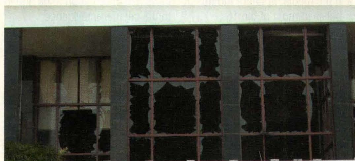
Damage is obvious at the Oberoi Restaurant, Mumbai
