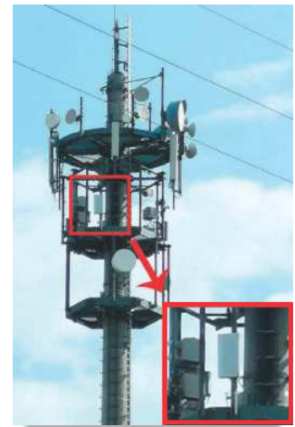
Cell phone mast already outfitted with 5G upgrade in Germany
